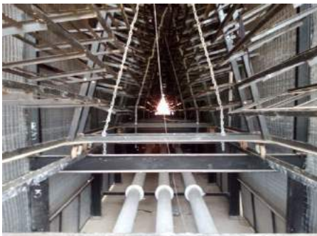
Figure 5: Trolley and heat pipe arrangement in the dryer
