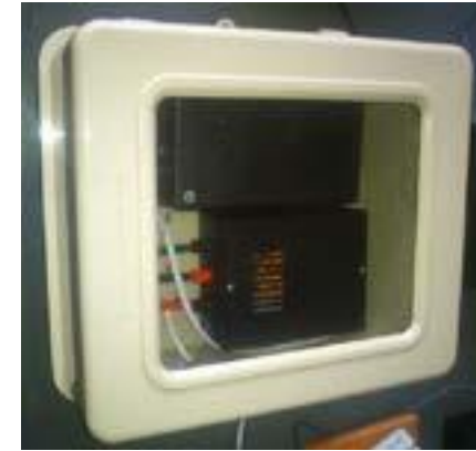
Figure 5: Controller unit inside the casing
