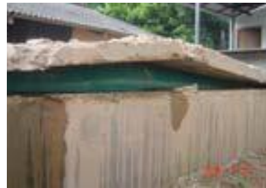
Figure 4: Top cover concrete slabs of the digester were raised up by the generated biogas
